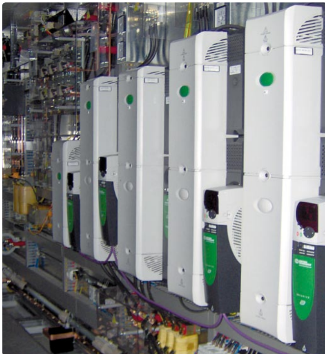
Typical crane automation system
