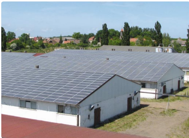
Kublank project, Meridian (Germany)
